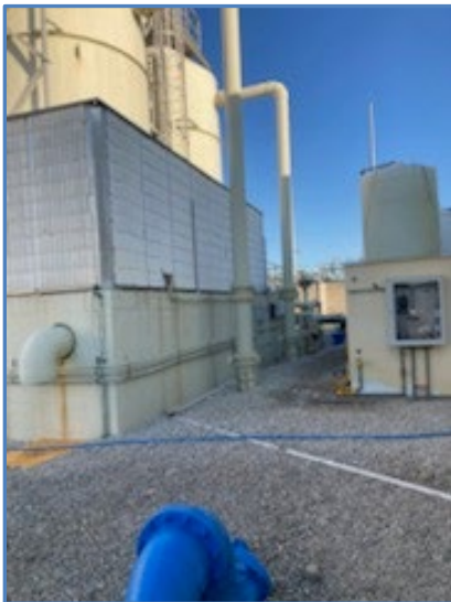
Replace Acoustic Wall
