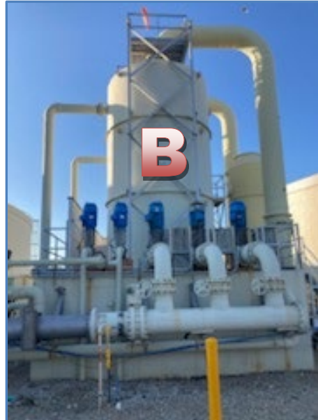
Front view of Degasifier B
